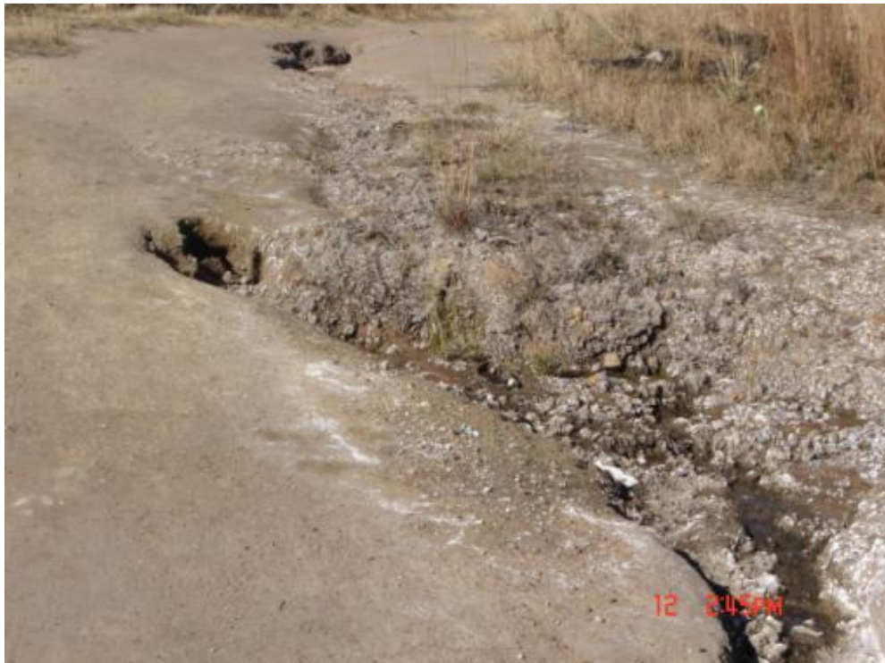
Photograph 14: Soil erosion taking place
